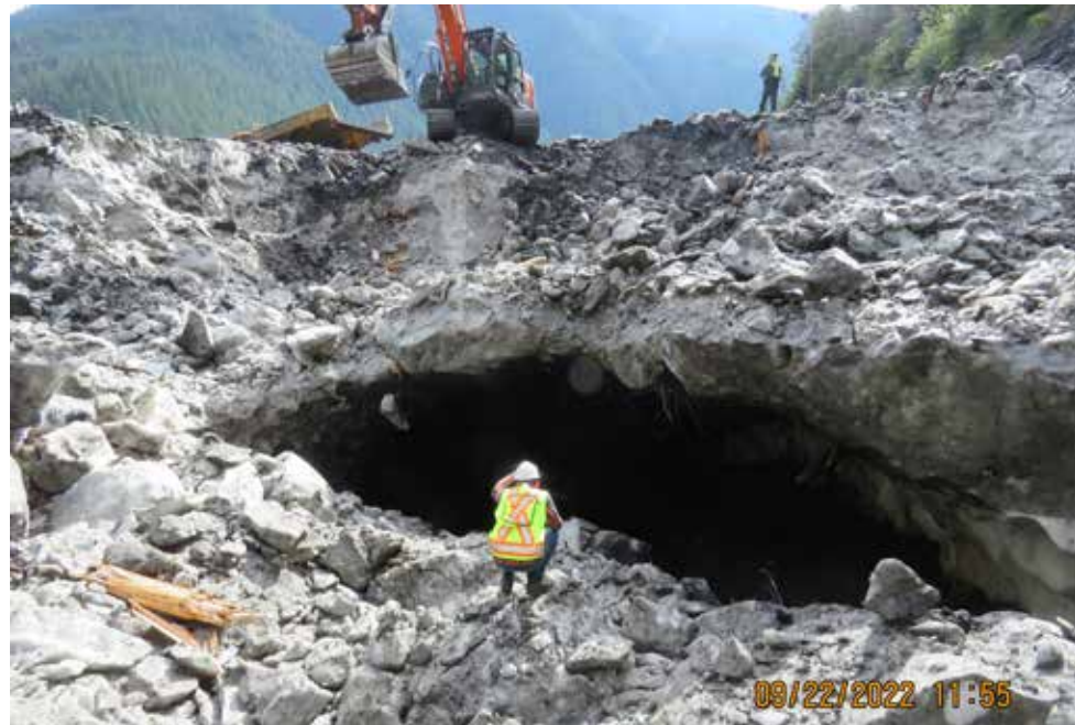
FIG. 8: SEPT. 22, 2022: CAREFUL WORK WAS REQUIRED REMOVING AVALANCHE DEBRIS DUE TO SNOW CAVE FORMATION ABOVE THE CREEK. THE EXCAVATOR IS APPROXIMATELY 15 M ABOVE THE ENTRANCE TO THE SHED'S DRAINAGE CULVERT.
