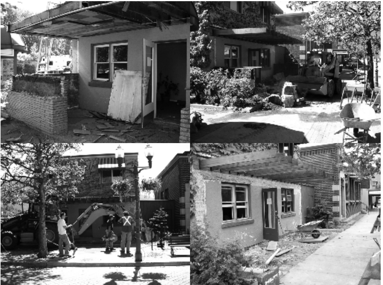
Going, going, GONE! It took contractors less than 2 days to remove the front of our building.
