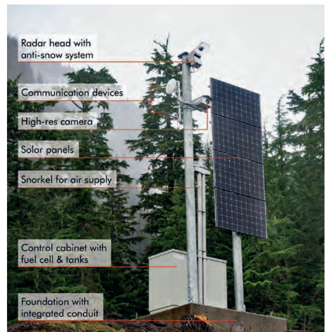
FIG. 3: AADS SYSTEM SETUP AT BEAR PASS.
