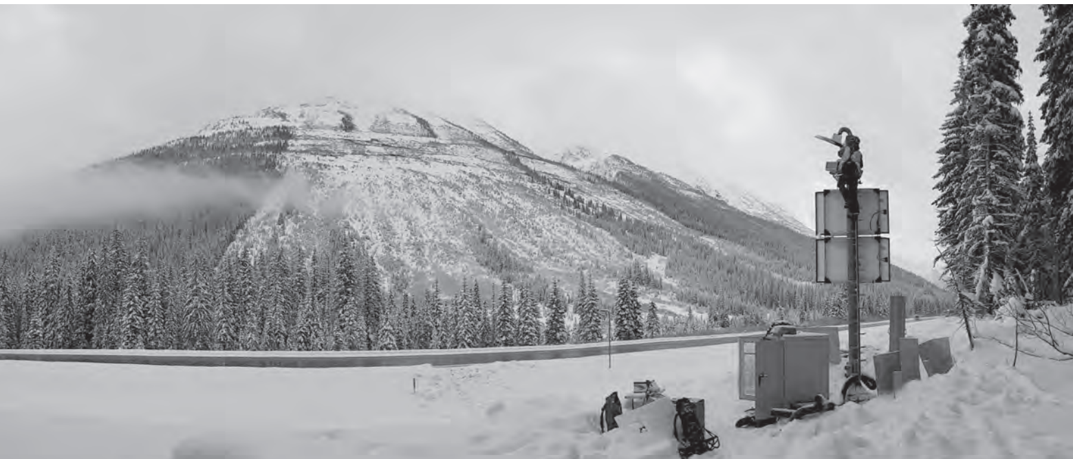
INSTALLATION OF THE DOPPLER RADAR AT THE MACDONALD WEST SHOULDER AVALANCHE PATHS // WYSSSEN CANADA
