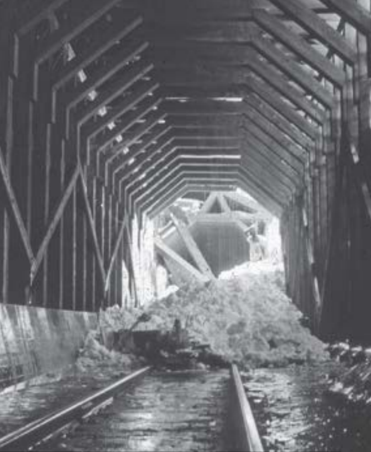
AN AVALANCHE DESTROYED PART OF A CPR SNOWSHED AT LAURIE SLIDE PATH WEST OF GLACIER NATIONAL PARK, BC, APRIL 1959 // REVELSTOKE MUSEUM AND ARCHIVES PETER SCHAEERER FOND PSS.38
